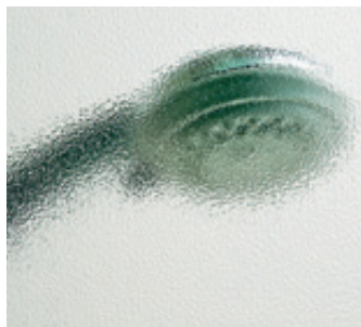
Detail of "arctic" design glass of the shower enclosure.
